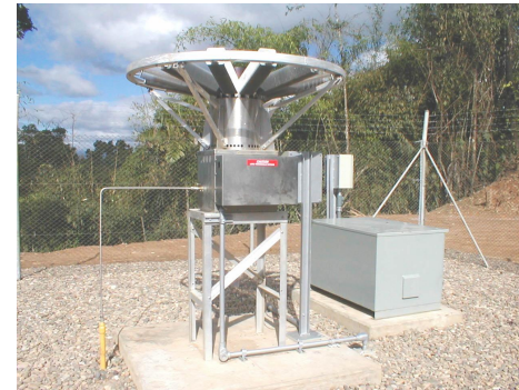
500 W TEG, natural gas pipeline, Peru [LeSage, Global Thermoelectric]
